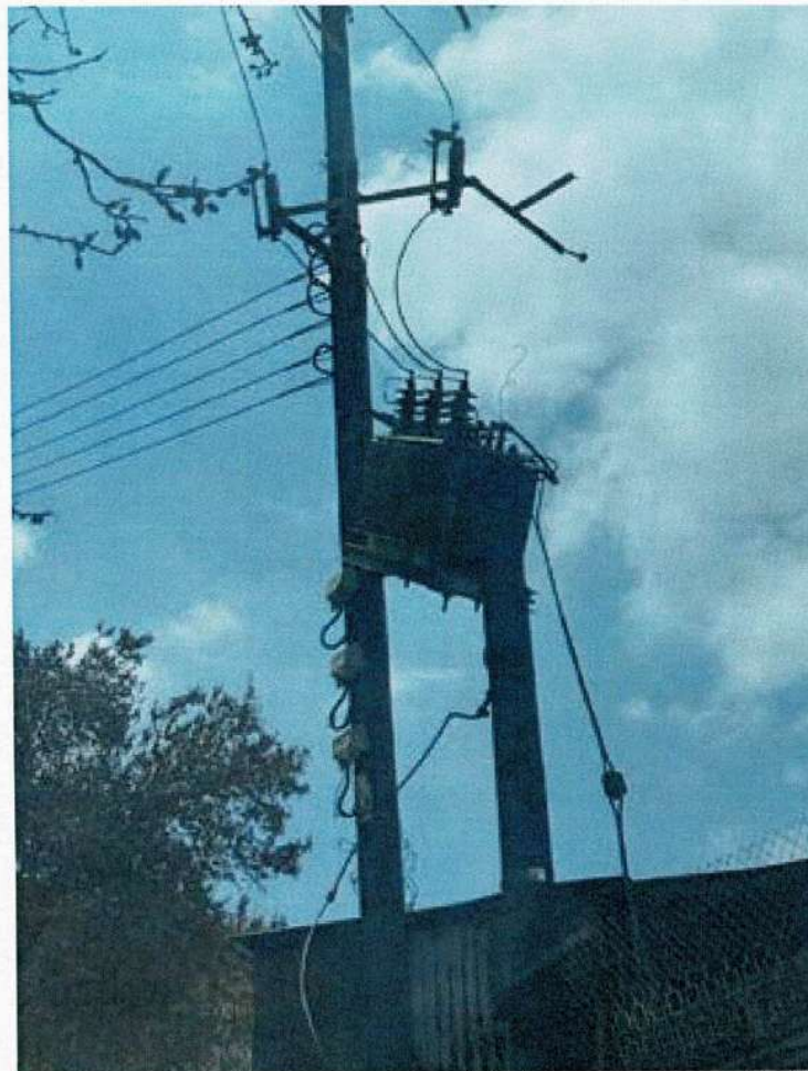
Figure 8: Example of fire damaged electrical infrastructure provided by EAC
