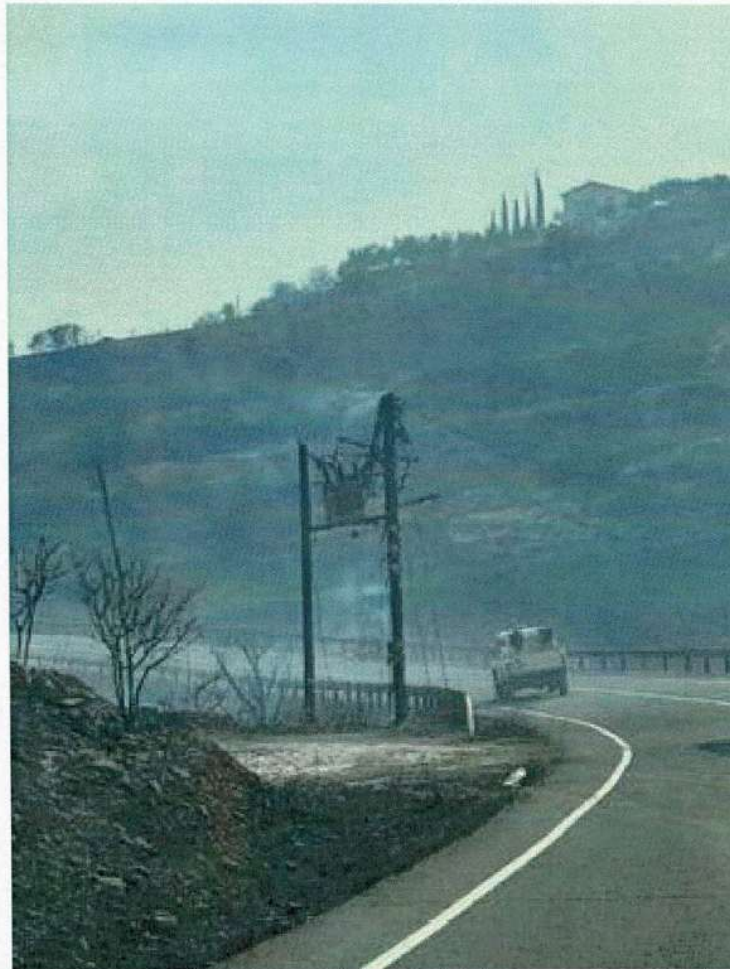
Figure 5: Example of fire damaged electrical infrastructure provided by EAC
