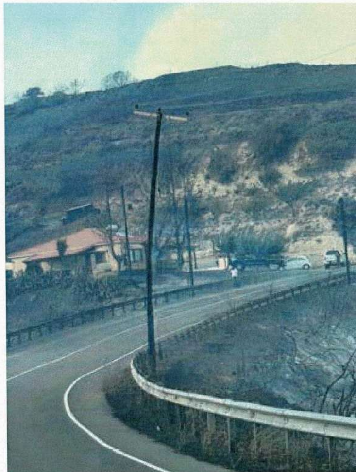
Figure 6: Example of fire damaged electrical infrastructure provided by EAC
